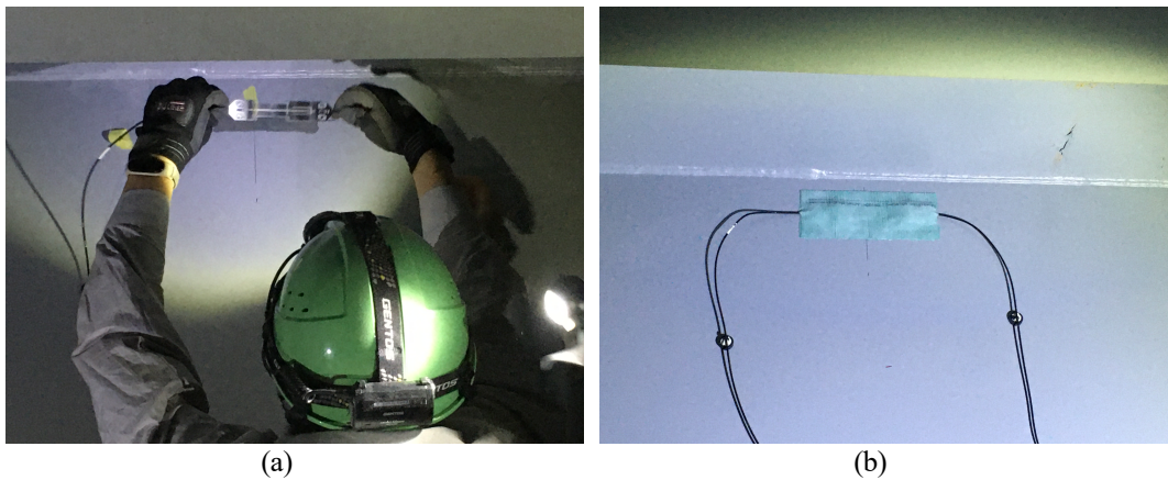
Figure 2. Fiber-optic strain sensor on the center girder: (a) Installation of the sensor; (b) Installed sensor.
